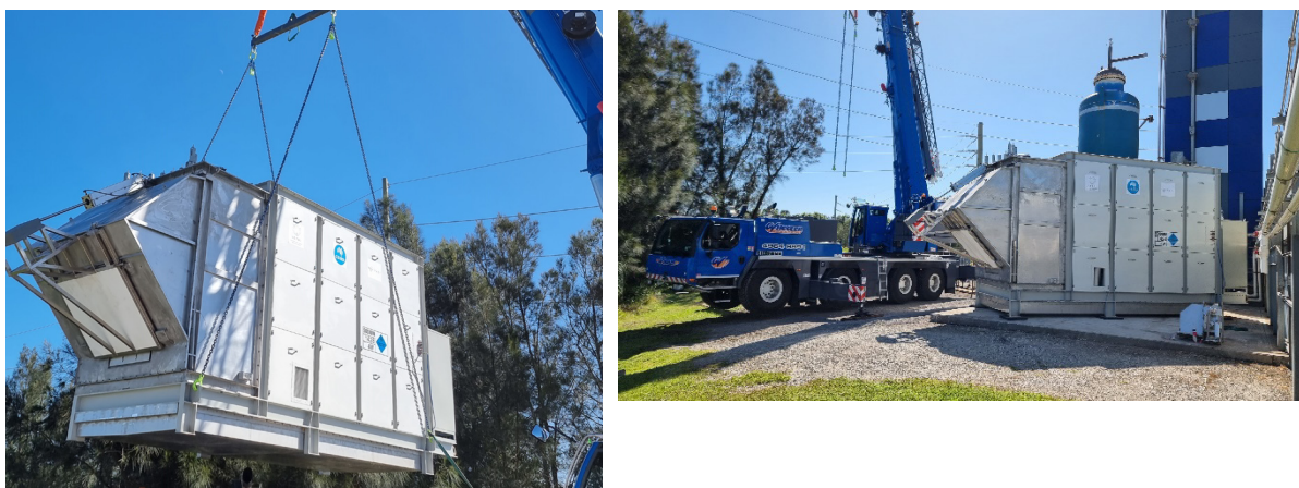
Figure 5 The main sodium module placed on its storage pad by crane at the base of solar tower 2.
