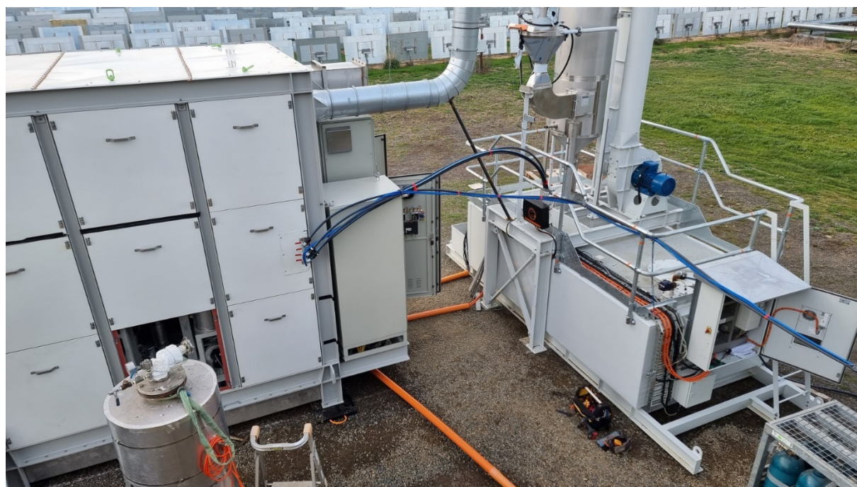
Figure 3 Both the sodium test loop module and wet venturi fume scrubber module connected together at Vast's Jemalong site.
