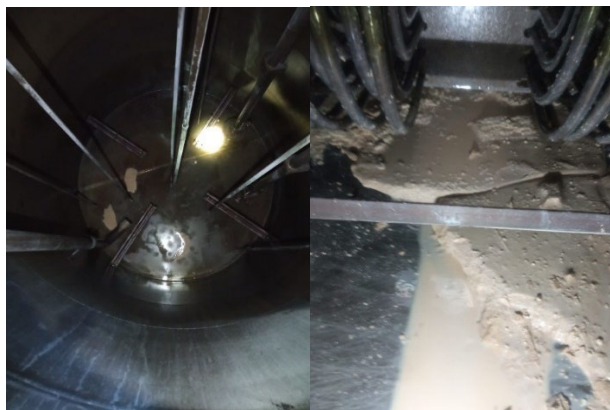
Figure 11. Left: Hot tank, right: Drainage tank.
