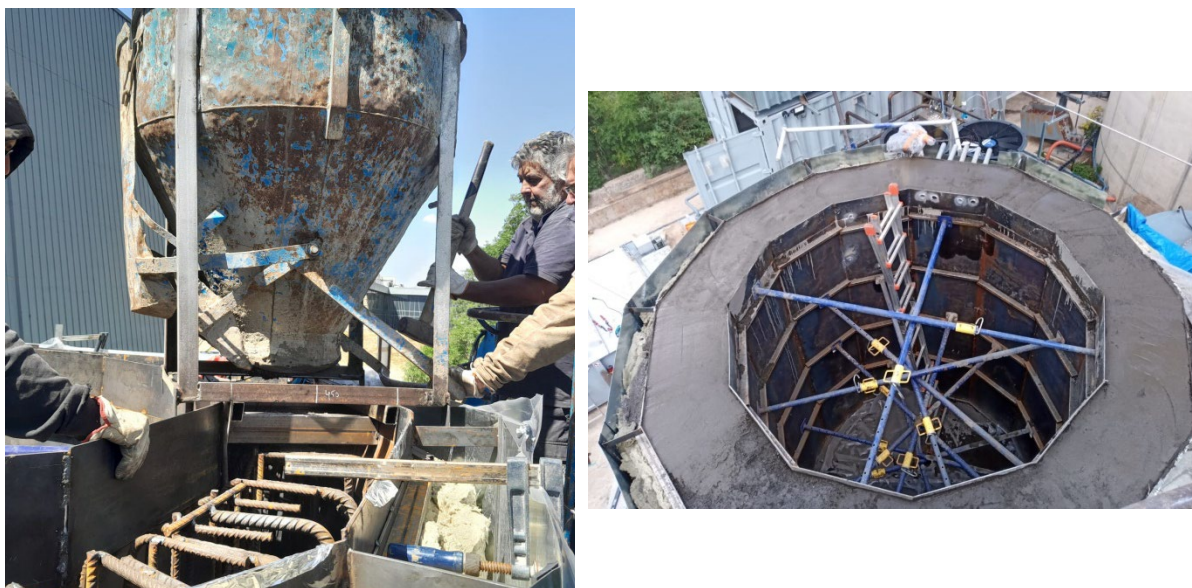
Figure 5. Manual pouring of concrete within the frame work and view from above of the tank with the concrete walls –blue rods kept the inner formwork at its position; they are removed after the concrete becomes complete cured and dry.
