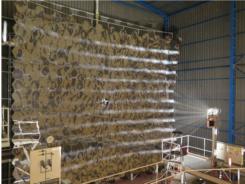
Figure 15. FAHEX100 concentrator in operation
