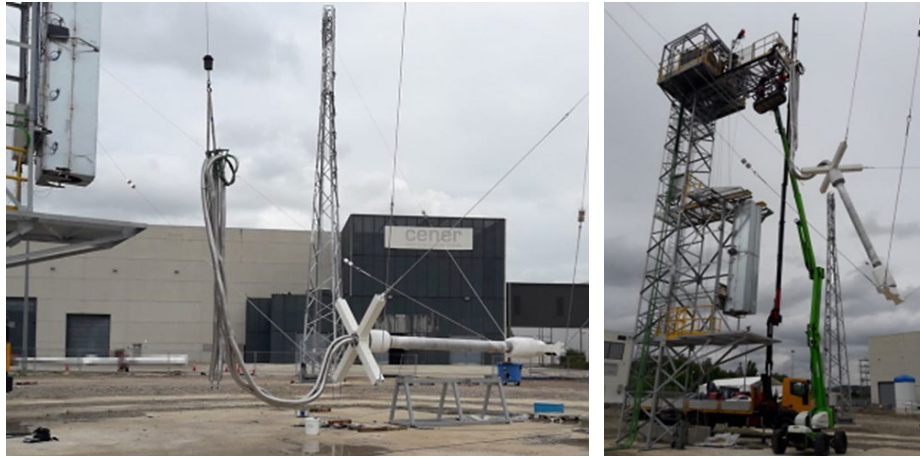
Figure 3. Receiver elevation process using the tracking system to bring it from the ground level (left) to the position in which the flexible hoses were soldered (right).
