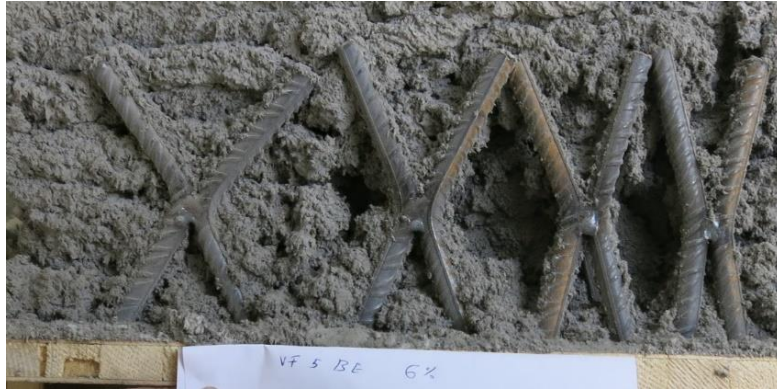
Figure 12: Resulting large cavities in test field 5 for accelerated material due to the shielding of material accumulated on the top surface.
