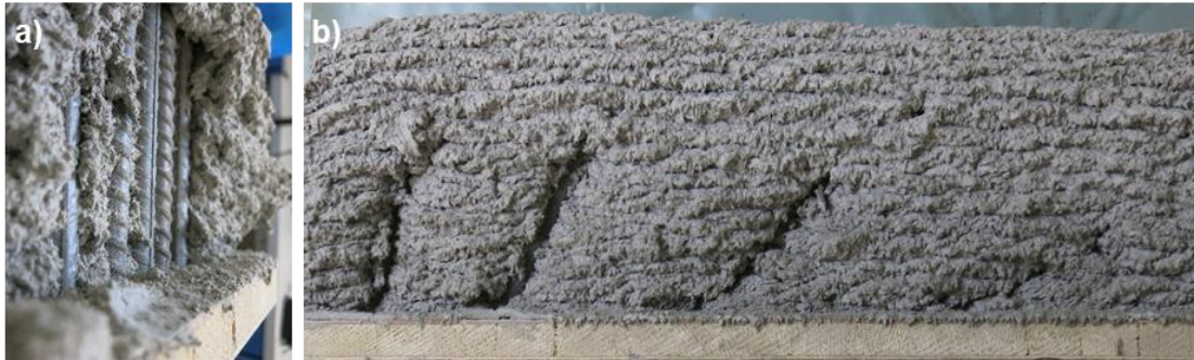
Figure 8: Lateral blocking of the unaccelerated material by reinforcement structure for a) test field 1 and b) test field 2.
