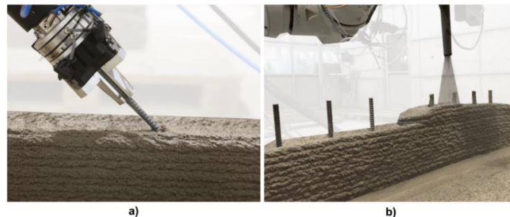
Figure 1: Process steps of short rebar insertion (SRI): a) angled short rebar insertion, b) enclosing process of protruding rebars.
