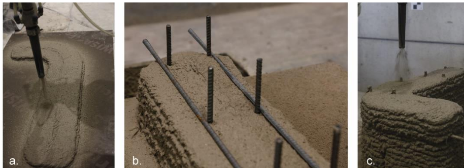
Figure 7. a) SC3DP process during first 150 mm segment b) integrated ILR and SRI after the first printed layer c) covering of integrated reinforcement and build-up of SC3DP layers
