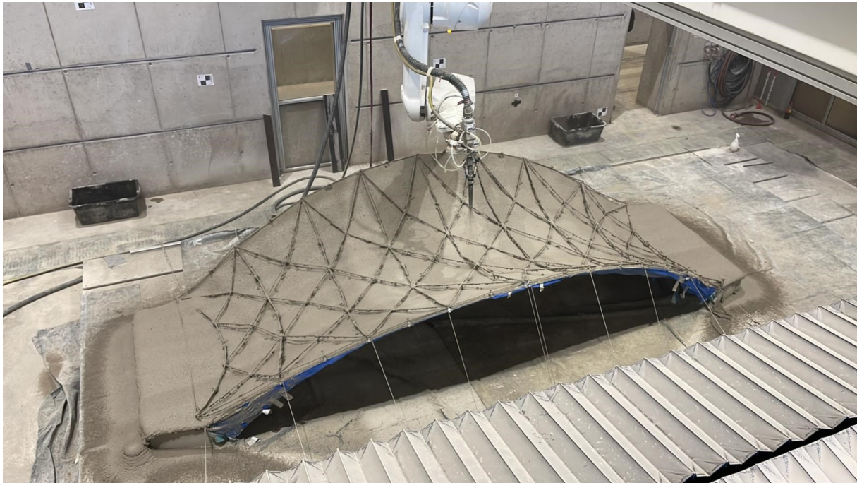
Figure 12. Exemplary application of the dynamic winding process: Robotically integrated fibre reinforcement as part of an additively manufactured pedestrian bridge
