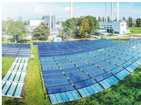
Figure 3. Image of the solar district heating plant Fernheizwerk located in Graz, Austria, showing one part of the installed collectors. Source: SOLID.
