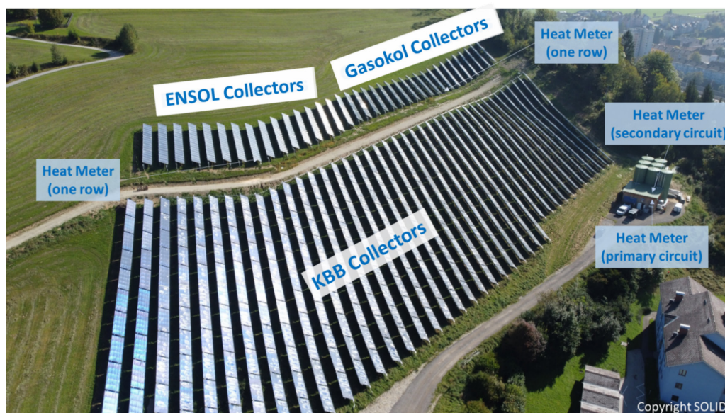
Figure 7: Picture of district heating plant in Mürzzuschlag showing the different collector fields and the installed heat meters. Source: SOLID.
