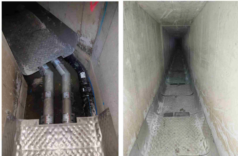
Figure 3: Installation of the heat exchangers in the sewer lines (Rabmer GreenTech GmbH/Uhrig).
