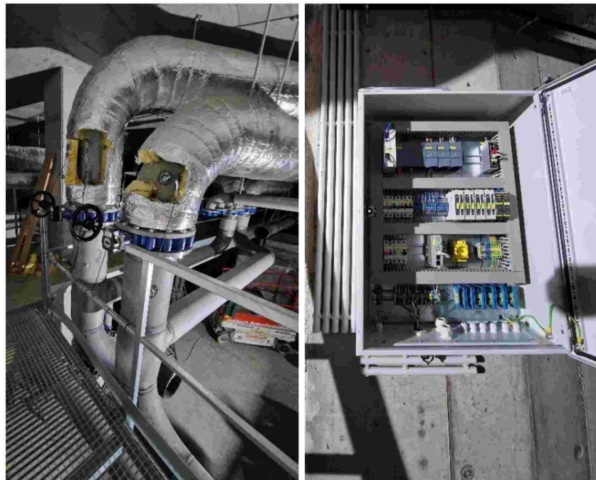
Figure 5: Installed sensors in the return and flow pipes to the heat pump (left) and the heart of the monitoring system: the switch cabinet (right) (Wiedemann, Rabmer GreenTech GmbH).
