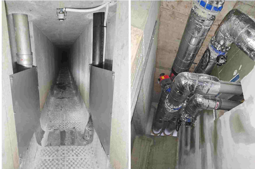
Figure 4: Installed monitoring sensor in the sewer (left) and return and flow pipes to the heat pump (right) (Rabmer GreenTech GmbH/Uhrig, Wiedemann).
