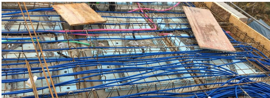
Figure 3. Picture of the multi-layer TABS during the construction process, the insulation layer shows gaps due to required reinforcement steel elements for stability of the ceiling
