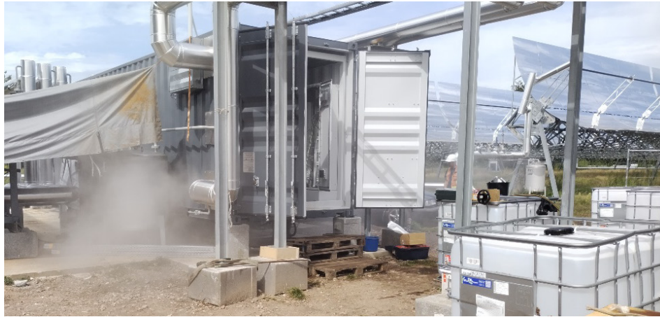
Figure 1. Blowing off air, water vapour and light gases from the collector circuit (Photo: DLR)
