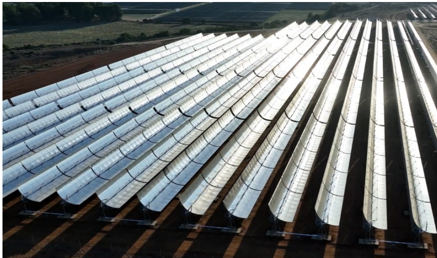
Figure 5. Western part of the solar field at Heineken Seville (Source: ENGIE [4])
