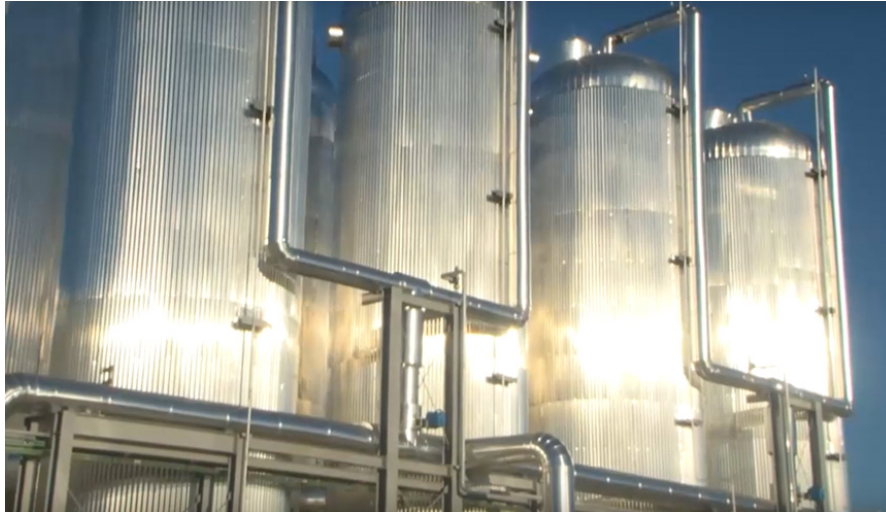
Figure 6. Pressurised water storage facility in Seville (Source: ENGIE)
